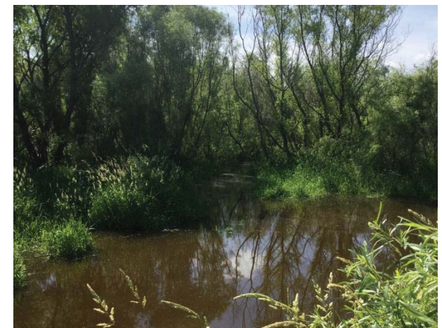
Dike along northern edge of property is breached and allowing consistent inflows from drainage ditch and Mauneshia River.
